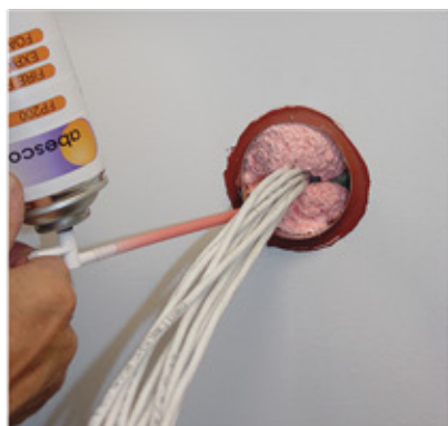
Cable Penetration Seals
